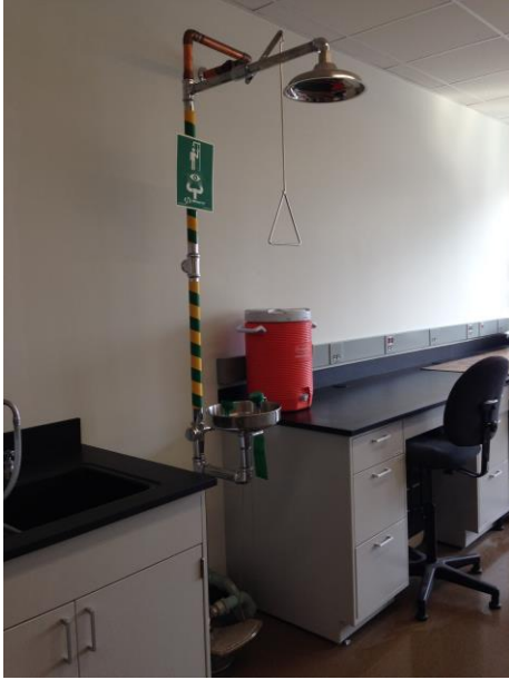
Figure 7: Shower & Eye Wash Station Room 245, South Side
