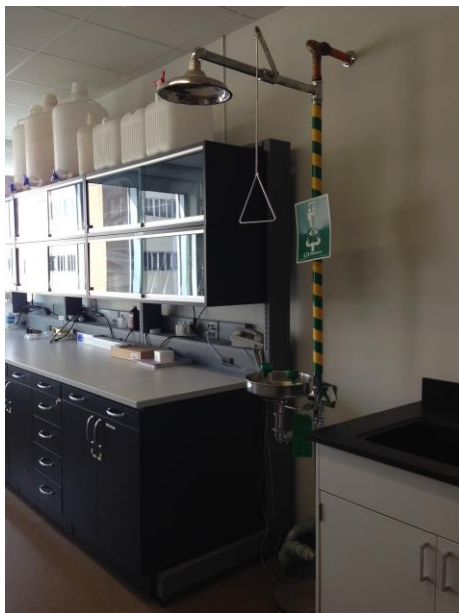
Figure 6: Shower & Eye Wash Station Room 245, North Side
