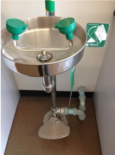
Figure 9: Shower & Eye Wash Station, Eye Wash Instructions
